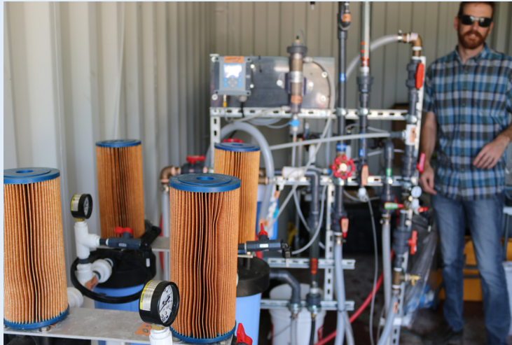
WCWC's on-site pilot installation included aeration, chlorination and filtration
