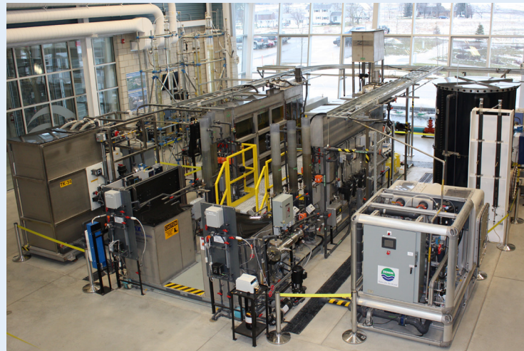
WCWC used their dual train, conventional pilot plant to compare chemical doses
